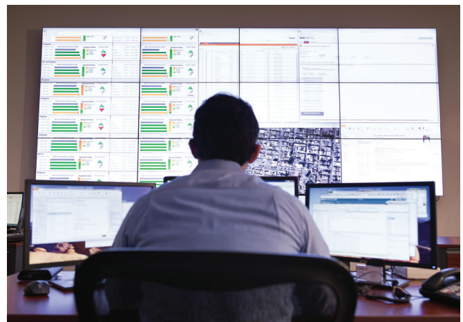
MUELLER NETWORK OPERATIONS CENTER IN ATLANTA, GEORGIA
